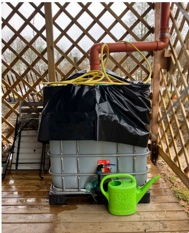
IBC tank at the farmhouse
